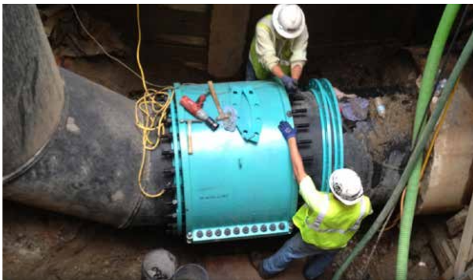
Ohio State University Chilled Water Line
